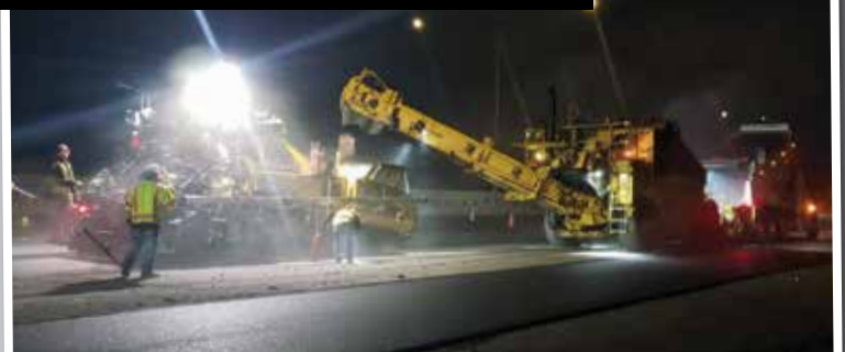
Members James Machado, Kevin Candelieri and Dominique Jackson work on I-880 for Bay Cities Paving and Grading.
