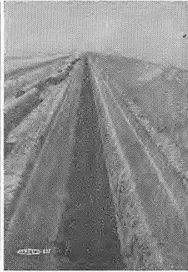
DEAD MAN'S LAKE near Twenty-Nine Palms was the site of this neat trenching job done by Operating Engineers with a 31 Parson Trenching Machine, Operator, Bob Burns. It's a good study in perspective and straight lines. ★ ★ ★
