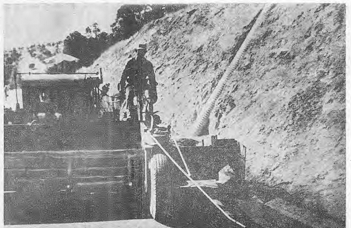
ABSCO PAVING has developed a new gadget for hot stuff. The extension on the right saves time in laying the shoulders. Vic Henry, with
