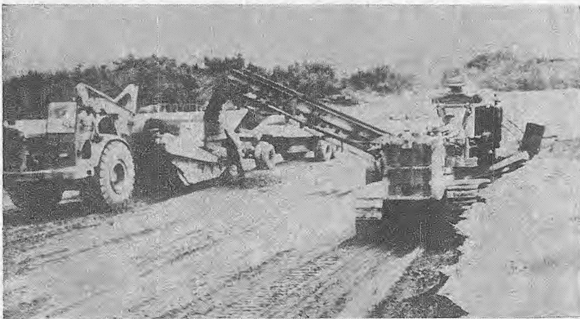
PRODUCTION is up on the Clifford C. Bong, Fortuna by-pass job. Here is why: A Sierra loader behind a D-8 cat, loading a DW 21 and bottom dump trailer. All material goes over the scales with a 70-ton pay load. There
