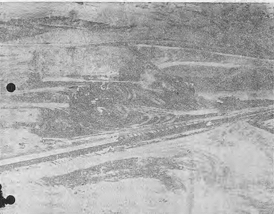
ADONNA Construction Company at the Hernandez Dam is getting well under way with approximately 30 Engineers on the job. Brother Harold
